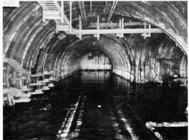
Another flooded tunnel shot, in Launcher Area 3. The original framing from the raised floor is visible below the water. The actual tunnel floor was 4-5 feet below the raised floor level
